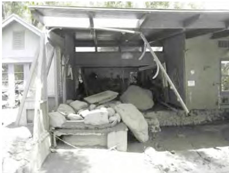
Home destroyed along Oak Creek
